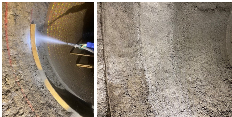
Almost dust-free gunning of REFKO Recovery MG (left) and repair zone after installation (right).
