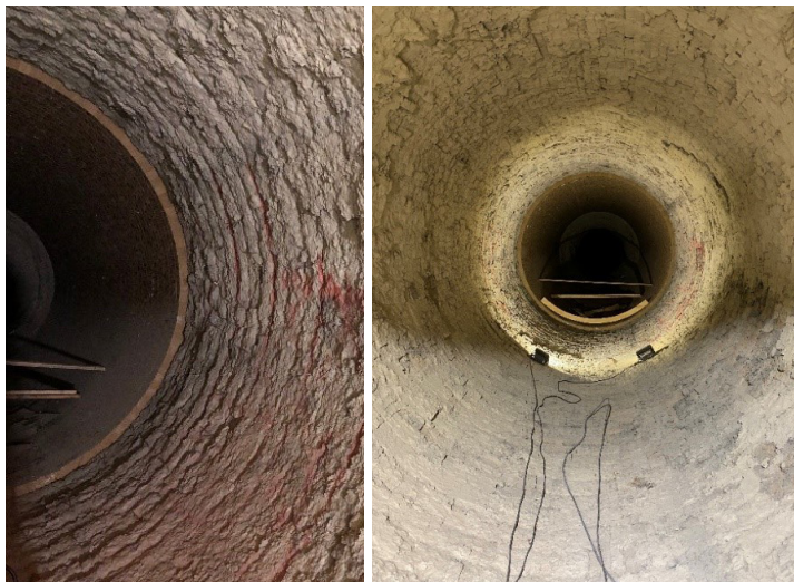
Premature wear of MgO/Spinel bricks.
